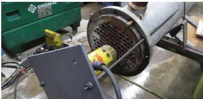
TUBE BUNDLE REMOVAL FOR REPAIR OR SERVICE
